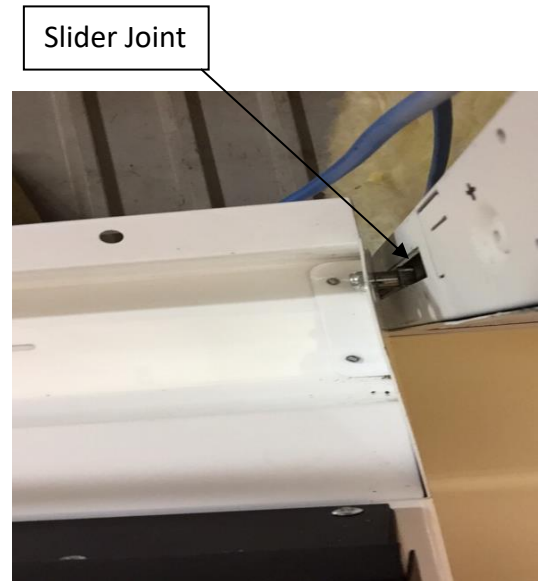
Figure 10: Fixture Hanging from Ceiling
